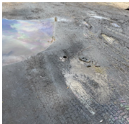
Leaking Underground Storage Tank
